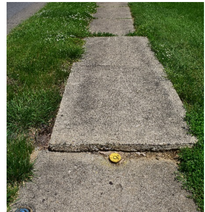
This segment of sidewalk along 21st Street has shifted and creates a hazard for users
